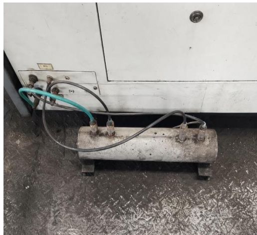
Gambar 5. Pergantian auto drain
